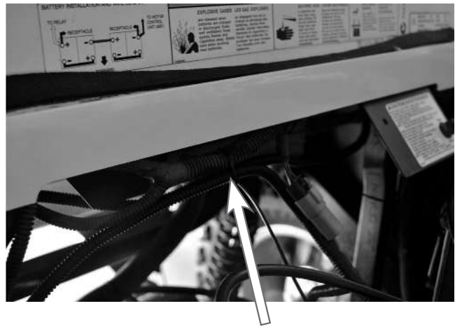
Zip tie to main harness at rear of battery compartment.
